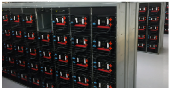
Example of a Multi MWH lithium energy storage system
