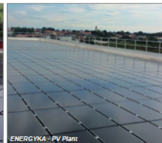
ENERGYKA - PV Plant 115KW in Udine, Italy
