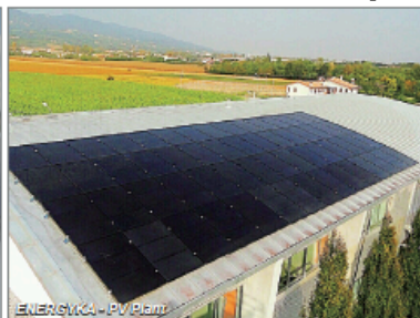
ENERGYKA - PV Plant 20KW in Asolo, Italy
